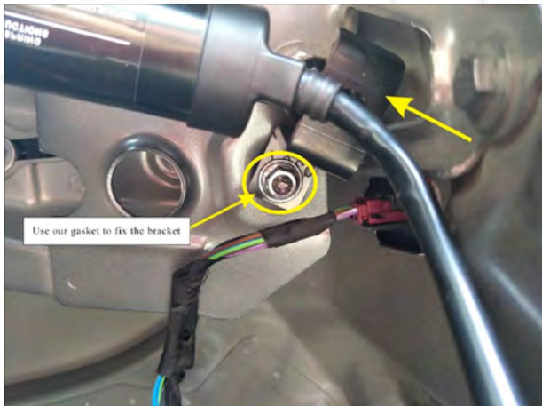
7. Remove the original car spring. Install our right bracket and brace rod, add a gasket on the hole of the bracket.
